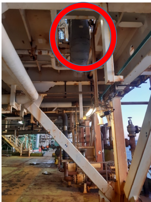
Figure 1- Shows the hole where the helmet dropped and the deck area below
