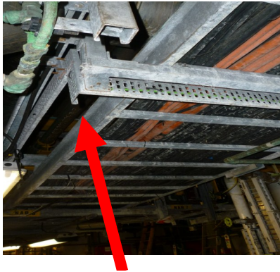
Cable Tray where Stilsons dropped from
