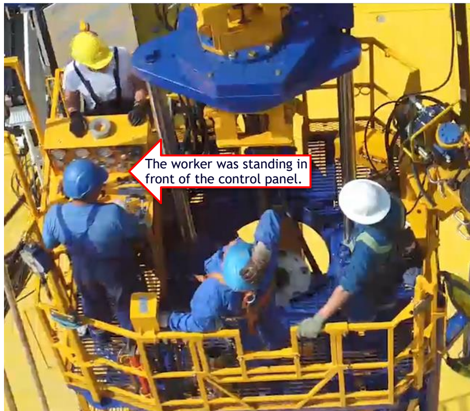
TYPICAL SET-UP OF A WORK PLATFORM ON A SNUBBING RIG. THE WORKER WAS STANDING IN FRONT OF THE CONTROL PANEL WHEN THE INCIDENT OCCURRED.
