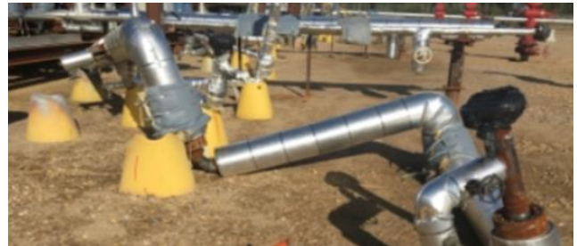
Example of pipe cone with dropped pipe section
