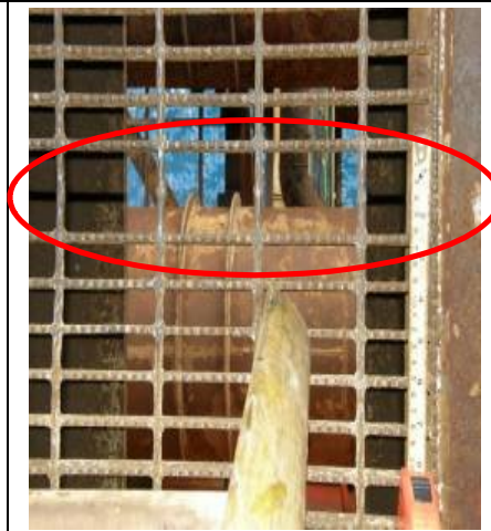
Gap in grating
